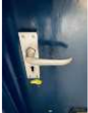
Non-compliant door handles
